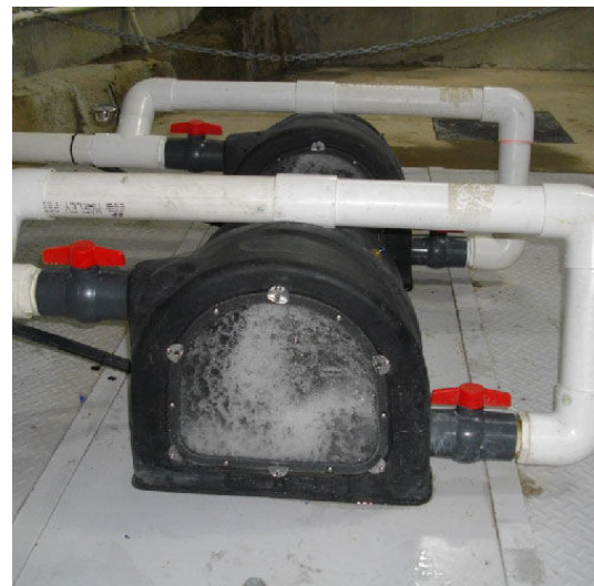
Manifold assembled on turbine
